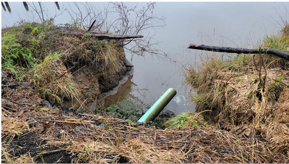
Figure 3-2: Sink Hole Around Pipe Following the NFS's 2024 Emergency Project.
