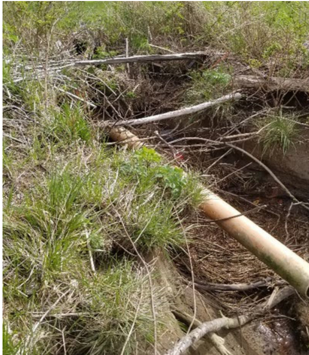
Figure 3-1: Undermined Outfall Pipe
